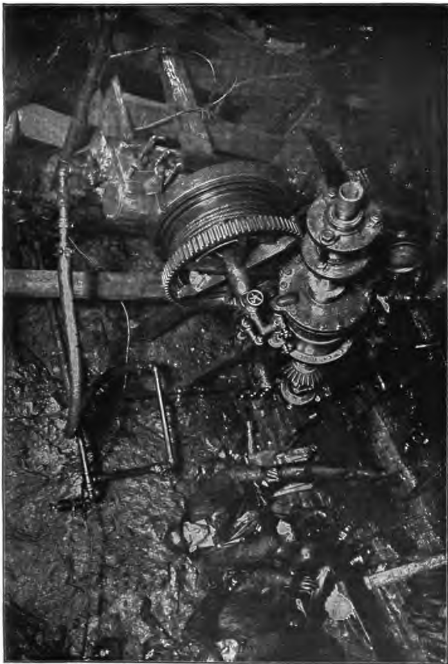
PLATE 24.—Hydraulic Diamond Drill at Work in Chamber of Test Shaft, Hudson River Siphon.
